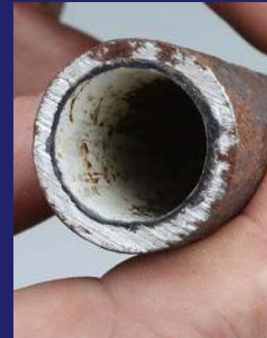
Lead-Lined Iron Service Line
